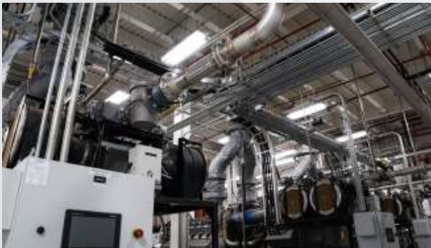
Bottler/Distillery | 8MW | Natural Gas
