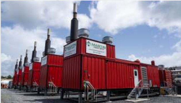
Bottling Plant | 6.6 MW | Propane
