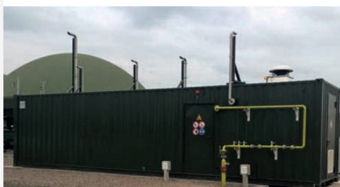
Biogas: 1,000 Nm 3 /hr Biomethane: 550-Nm 3 /hr
