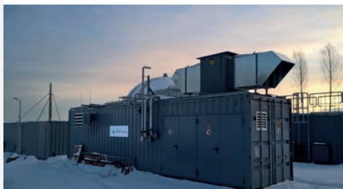
Biogas: 100 Nm 3 /hr Biomethane: 55 Nm 3 /hr
