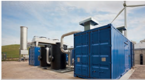
Biogas: 1,000 Nm 3 /hr Biomethane: 620 Nm 3 /hr
