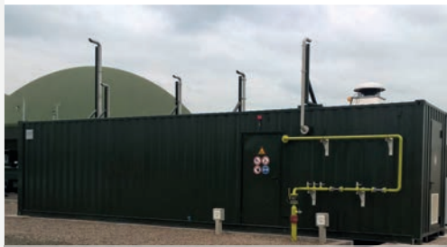
Biogas: 1,000 Nm 3 /hr Biomethane: 550-Nm 3 /hr
