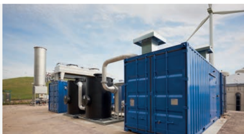
Biogas: 1,000 Nm 3 /hr Biomethane: 620 Nm 3 /hr
